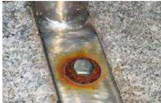
Figure 3 Standard case of contact corrosion
