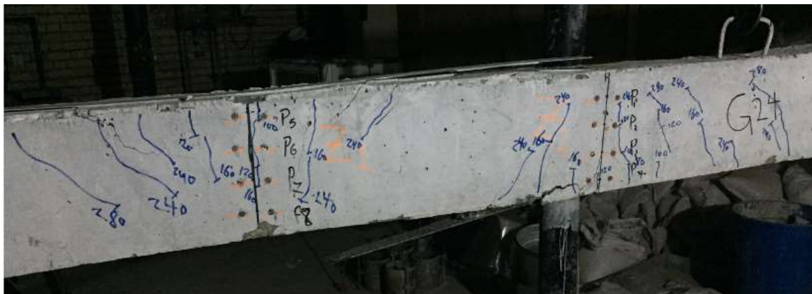
Figure 17 The patterns crack of beam G24.
