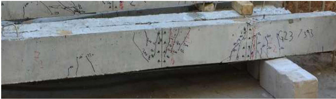
Figure 16 The patterns crack of beam G23.
