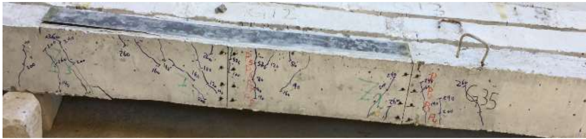
Figure 23 The patterns crack of beam G35.
