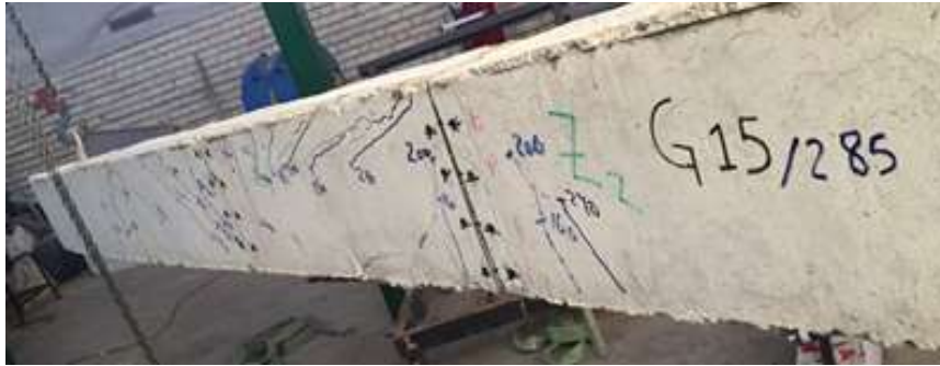
Figure 13 The patterns crack of beam G15.
