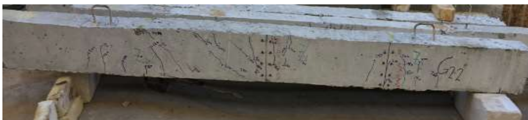
Figure 15 The patterns crack of beam G22.
