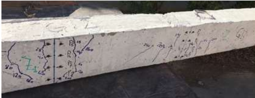
Figure 11 The patterns crack of beam G13.
