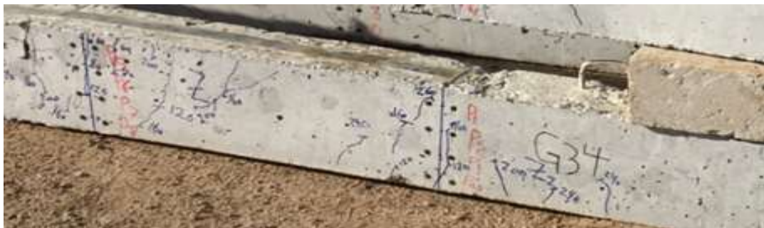
Figure 22 The patterns crack of beam G34.
