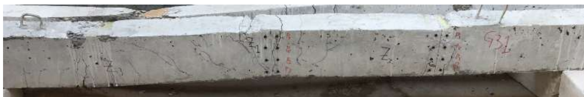
Figure 19 The patterns crack of beam G31.
