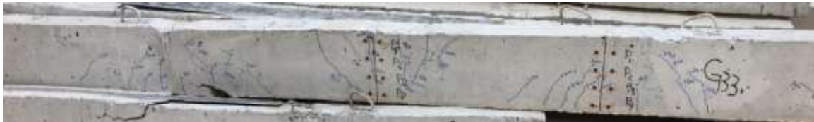
Figure 21 The patterns crack of beam G33.
